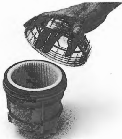
Controle koelwaterfilter. Checking raw water strainer.
